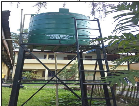
Photo 3: Arsenic removal water plant for detoxification
