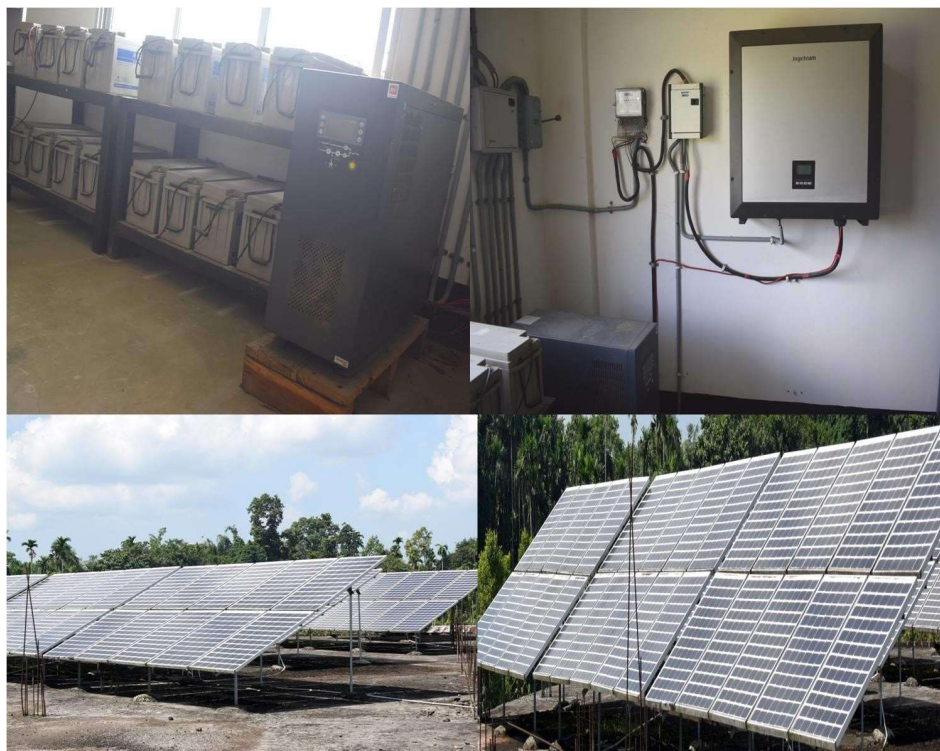
Photo 20: Solar panel system in the college building and related infrastructure
