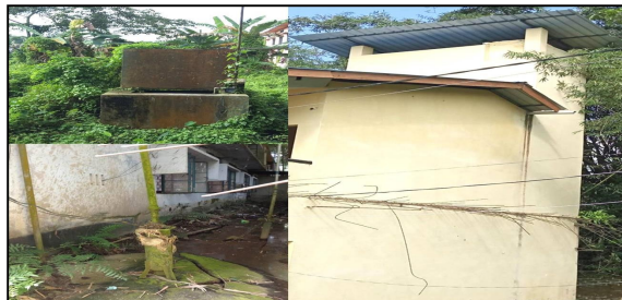
Photo 2: Water supply system in the college campus
